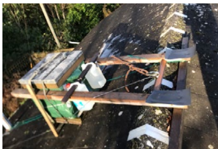
An eye bolt goes through the roof with a nut on the inside.
