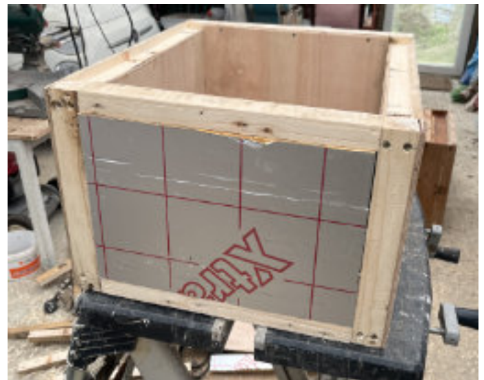
First step – make the inner frames and place two layer of insulation in the empty space. The inner walls are 5.5 mm plywood.
